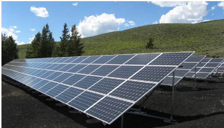
Figure 18. A ground mounted solar energy system. 119
