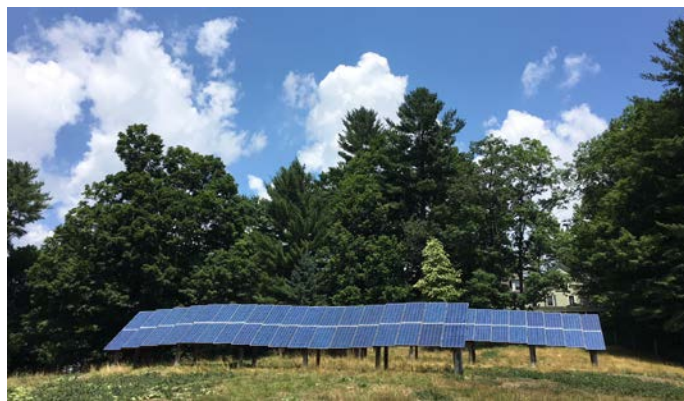
Figure 4. A ground mounted solar energy system in Brattleboro, Vermont.
