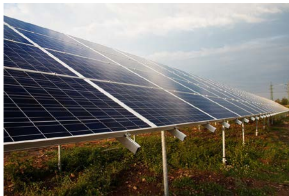
Figure 11. Solar panels in a field. 79
