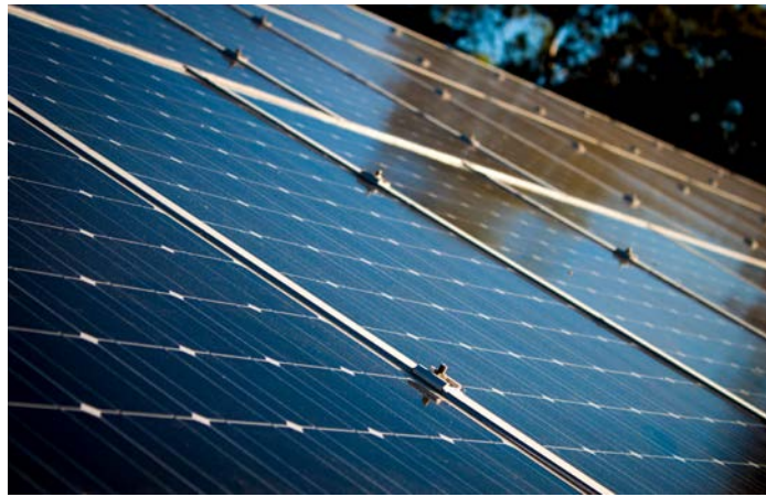
Figure 9. Close up of PV panels. 56
