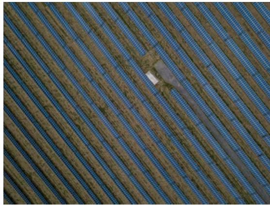
Figure 7. A large scale ground mounted solar energy system. 29
