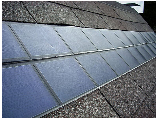
Figure 12. Integrated solar system in Louisville, Kentucky. 83
