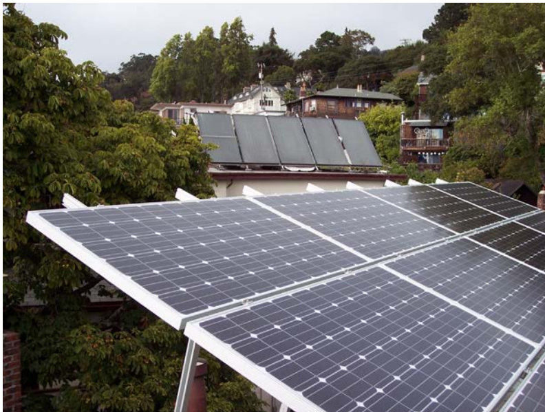
Figure 10. Solar panels located within a residential area. 75
