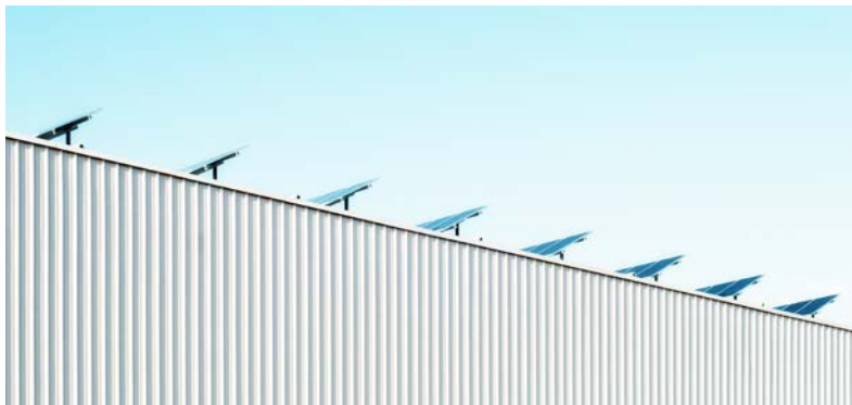
Figure 16. Angled rooftop solar panels on a flat roof visible from the ground. 104
