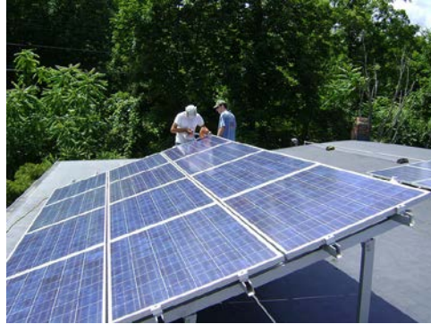
Figure 17. Angled solar panels on a flat roof. 117
