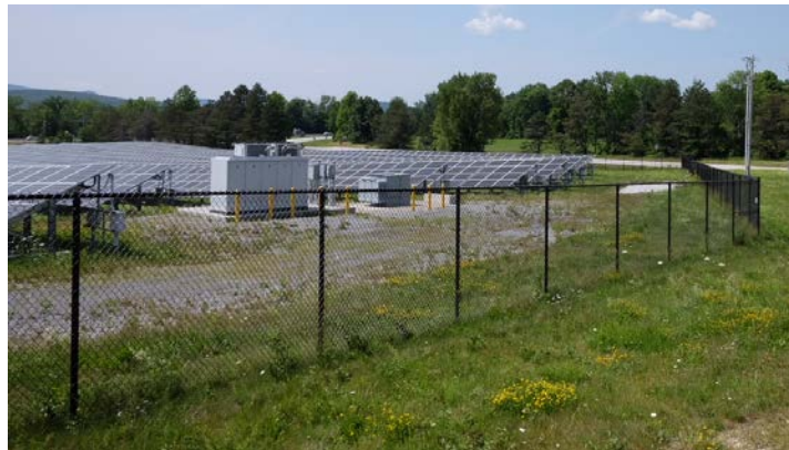
Figure 21. The Clarendon Solar Farm in Vermont with no visual buffer but with a security fence.
