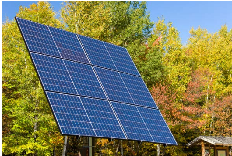
Figure 13. Trees and solar panels functioning in proximity. 90
