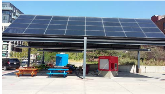
Figure 5. Solar canopies overlaying outdoor seating and garage. 20
